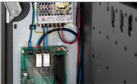
Cabling according to VDE guidelines
